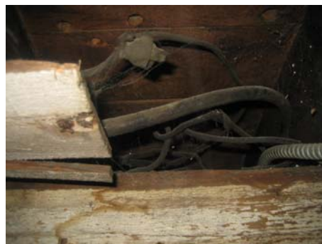
Live knob and tube wiring found in one of several areas in basement
