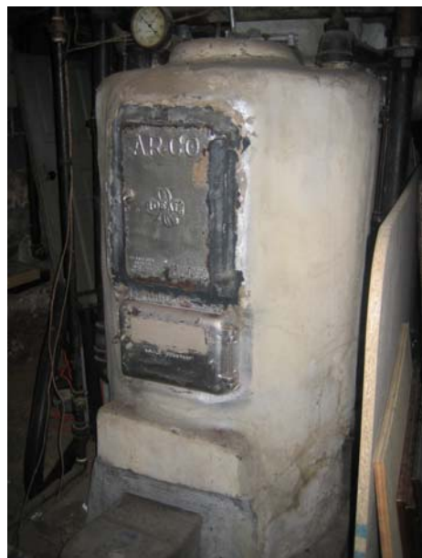
Old boiler, wrapped in an asbestos like substance
