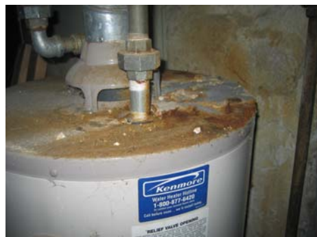
Corrosion on water heater appears to have been caused by an old leak from above.
