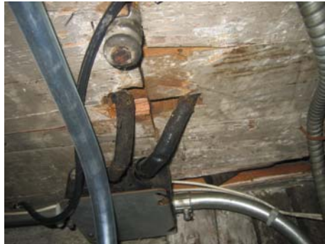
More knob and tube wiring found near electric panel
