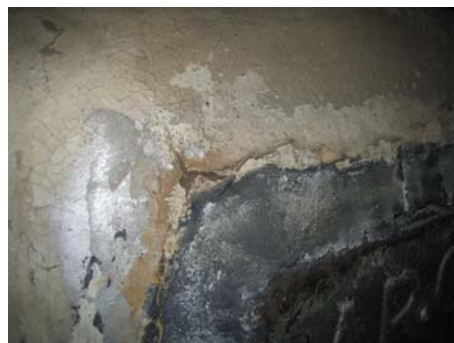
Edges of asbestos like substance are broken, making it possible for this substance to become air born.
